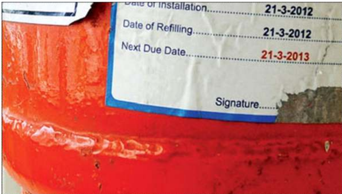
Fig 6.4.1.3 Know the refill date on the fire extinguisher
